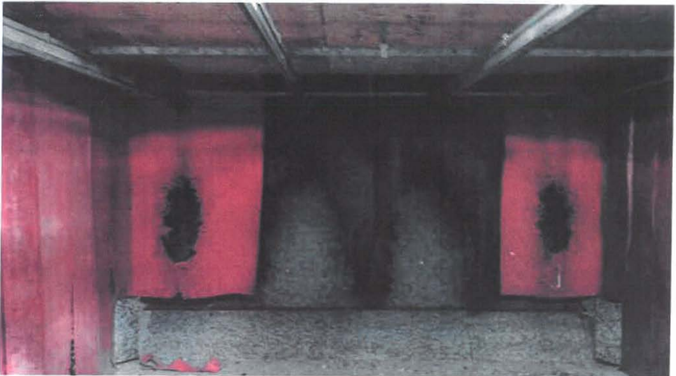
Sheet metal backstop, red rubber impact absorbing material, and plywood ceiling at target end of gun range
