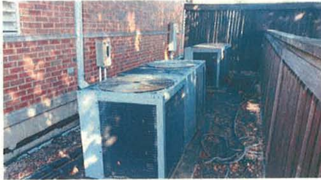
Condensing units for AHU-2 and AHU-3
