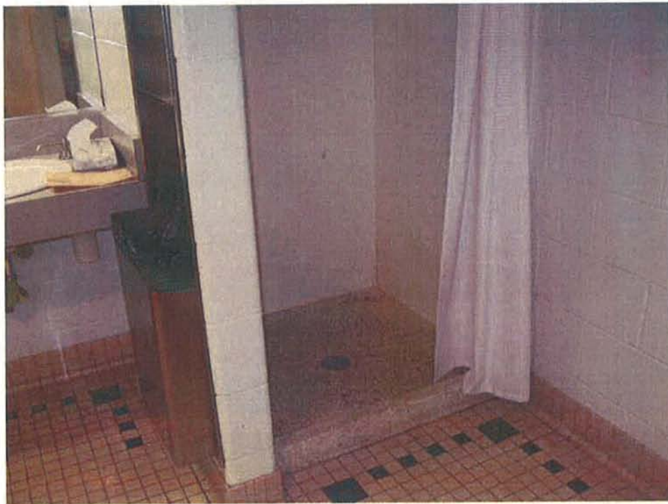
Showers with curbs are not accessible. One accessible shower stall for each sex is required.
