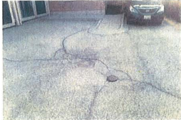
⑳ Looking northeast at the valve boxes in the employee lot.
