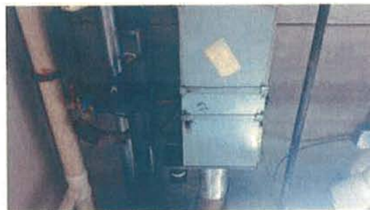
Typical vav box with hot water coil
