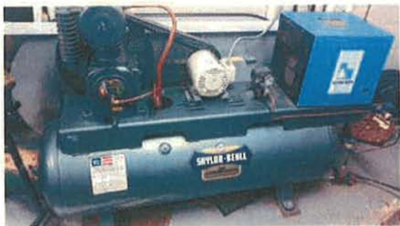
Air compressor for pneumatic controls
