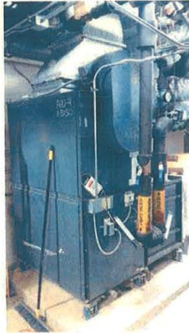
AHU-4 in basement
