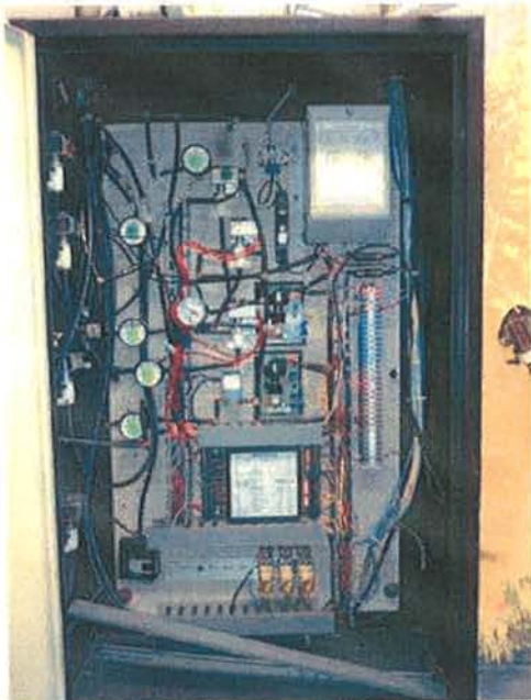
Pneumatic controls panel
