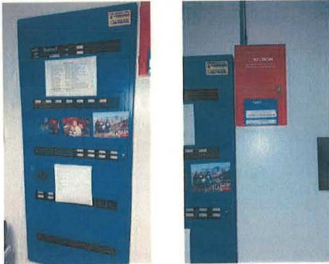
Fire Alarm Control Panel Keltron Wireless Transmitter
