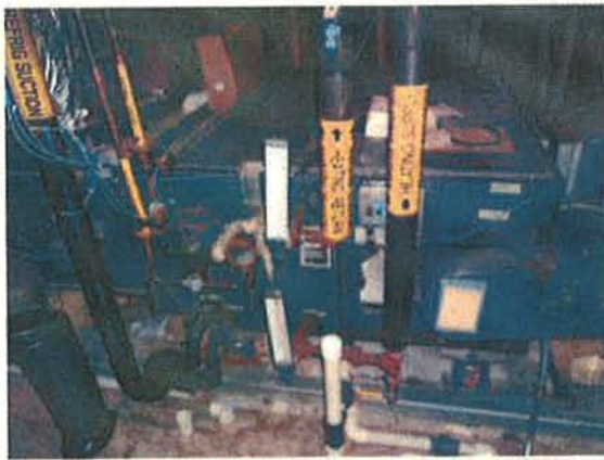
AHU-1 in attic, typical for AHU-2
