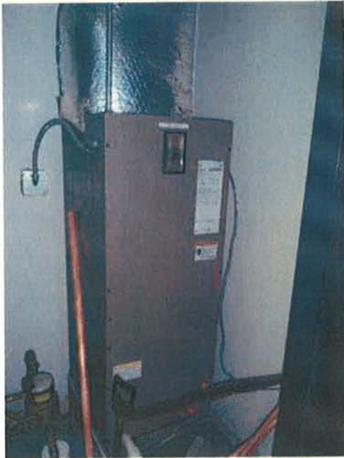
Electric furnace for remote garage
