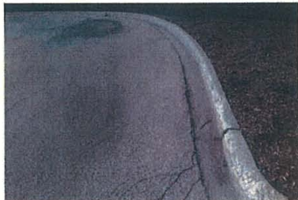
⑱ Looking east at the pavement in the employee lot.
