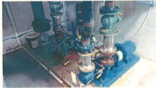
Hot water distribution pumps
