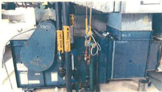
AHU-3 in basement
