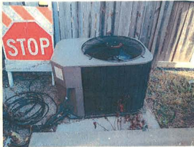
Condensing unit for remote garage
