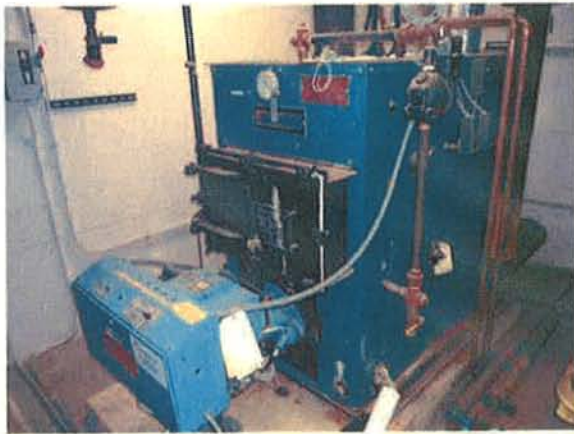
Heating boiler, typical for 2
