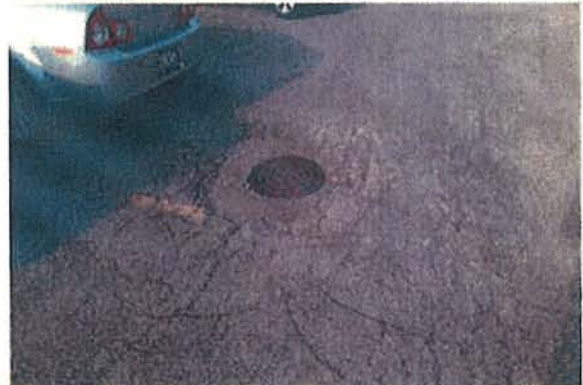
⑯ Looking at the pavement around a drainage structure in the employee lot.
