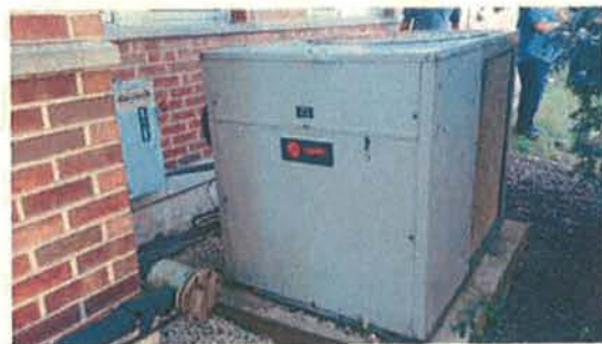
AHU-1 condensing unit (10 ton)
