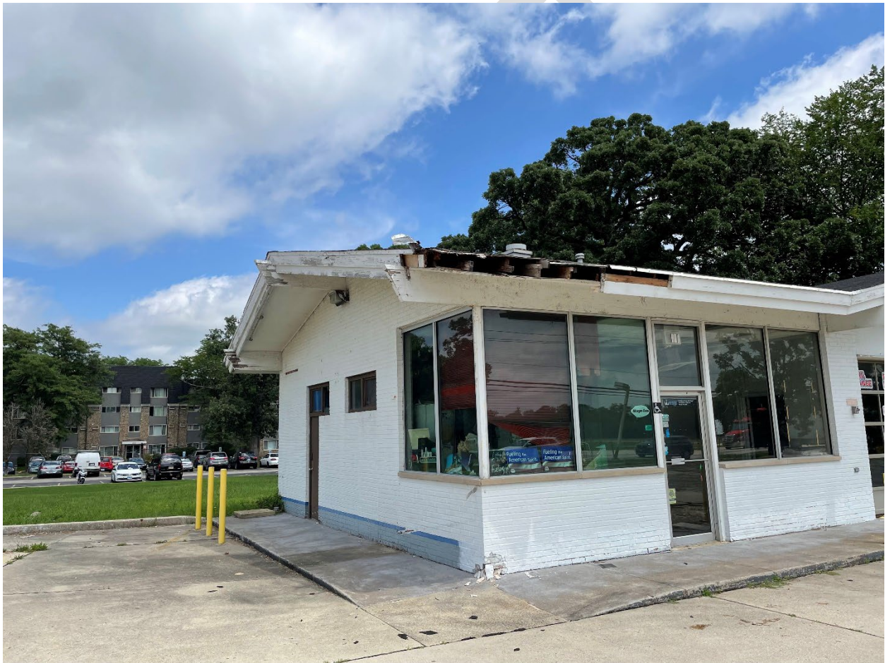
ABOVE: Example of Deterioration observed during field survey. Source: Teska Associates, Inc.
