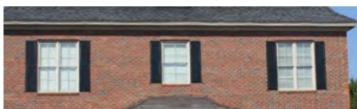
Inappropriately Scaled Shutters: Not Permitted
