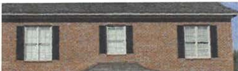
Inappropriately Scaled Shutters: Not Permitted
