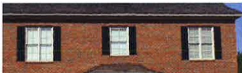
Inappropriately Scaled Shutters: Not Permitted
