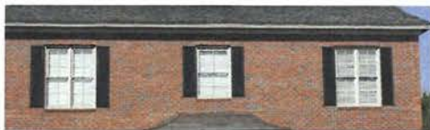
Inappropriately Scaled Shutters: Not Permitted
